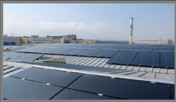
Commercial - Roof top
